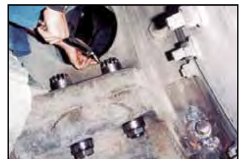
Split Gear segment on rotating kiln.
